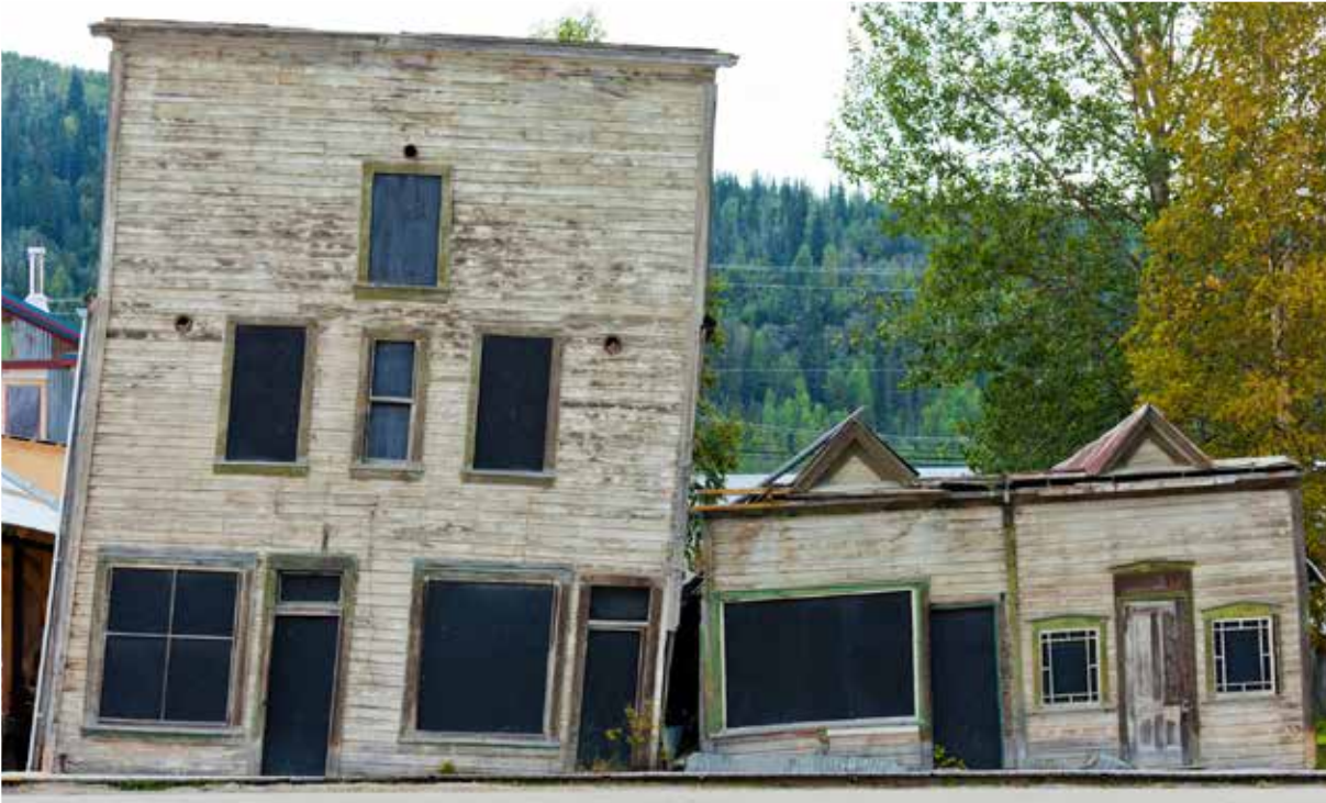
Melting permafrost has already cost cities like Dawson City, Yukon, hundreds of thousands of dollars—as buildings slant, pipes burst and roads crack, according to reports published by the CBC. PHOTO: PI-LENS/SHUTTERSTOCK
